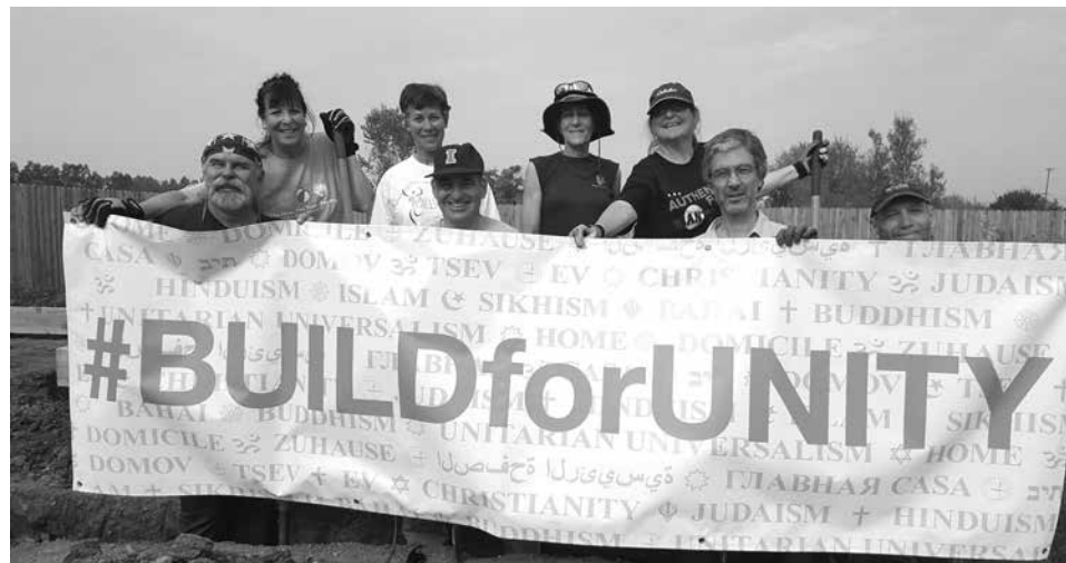
Congregation B’nai Israel members are joined by a Habitat for Humanity site supervisor as they contribute to building homes as part of the “Build for Unity” program.
